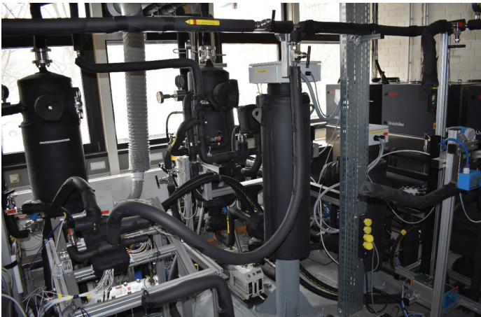
Figure 3. SCARLETT facility – testing of heat exchanger plates as part of the sCO 2 effort (photo: A. Wahl, IKE, University of Stuttgart)
